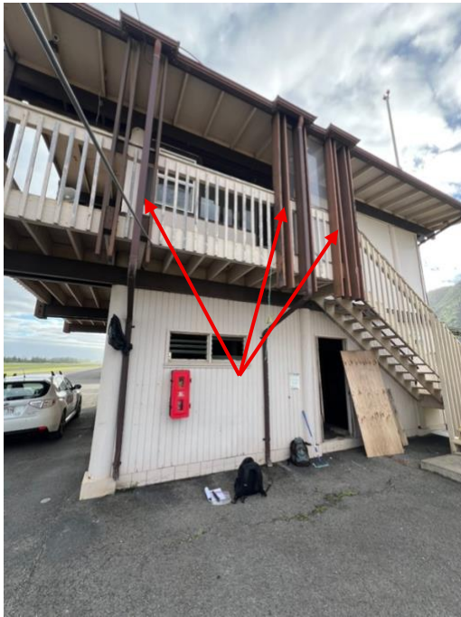
Lead-containing paint detected on exterior 2X6 Vertical Decorative Supports
